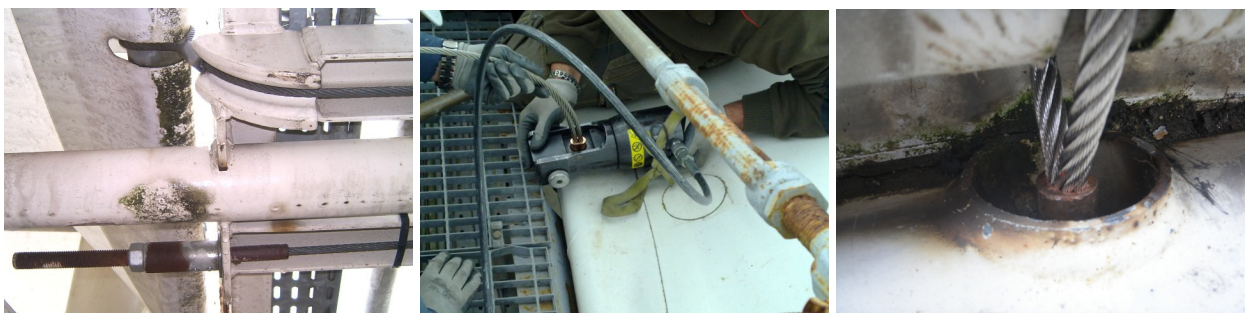
Figure 9: Corroded wire ropes, replacement with stainless steel wire ropes
